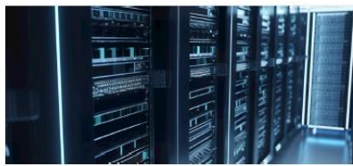
Power distribution package for datacenter of IT major
