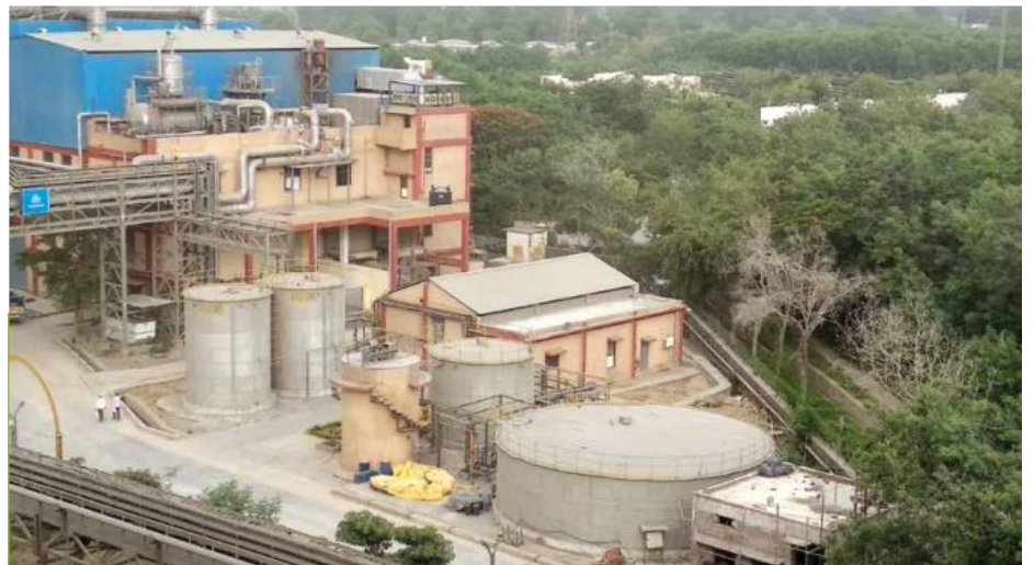
Figure 49: WHRS site at Satna in Madhya Pradesh - Boiler
